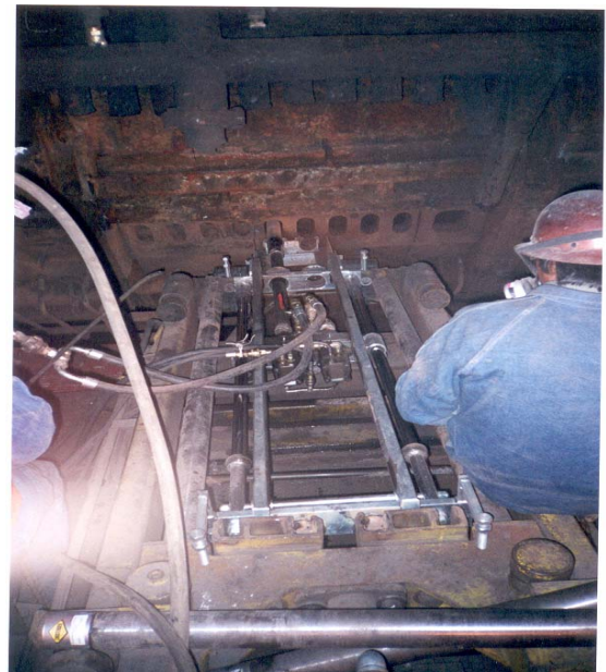
Dual Drill Heads mounted on Gase Tuyere Puncher
